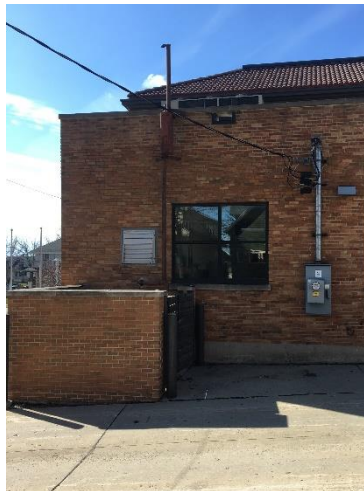
Service Entrance and Utility Meter Fire Administration Building
