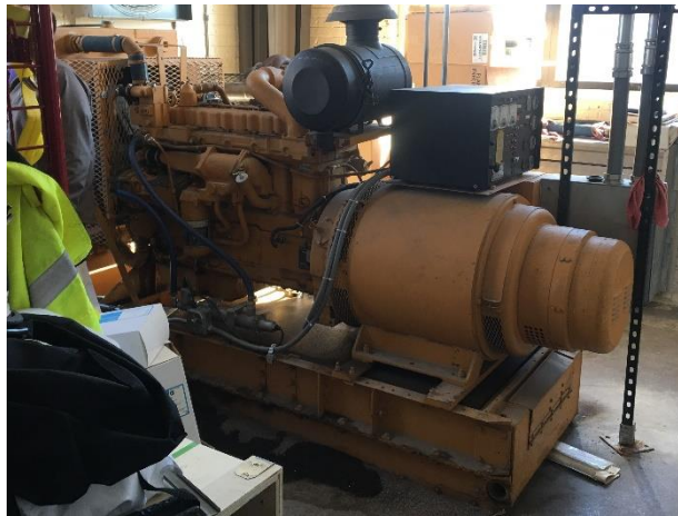
Existing Generator Located in Garage
