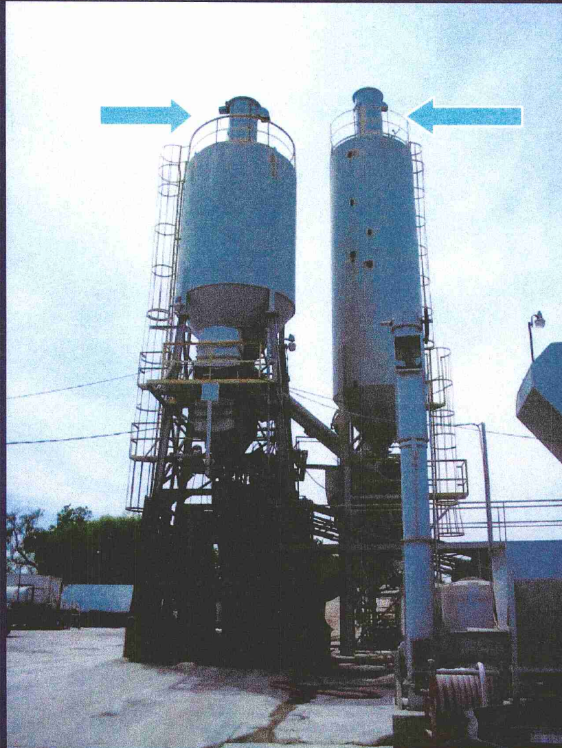
Baghouses on Cement/Fly Ash Silos
