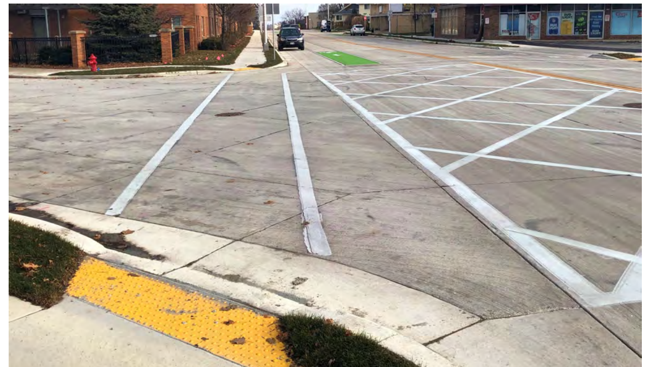
ADA compliant curb ramp at the intersection of W. Beloit Rd. & S. 67 th Pl.
