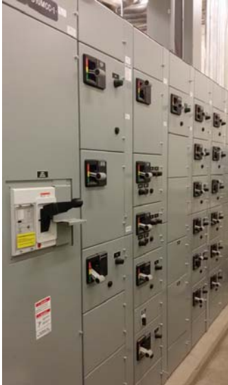
Energenecs Supplied MCC at Eau Claire WWTP
