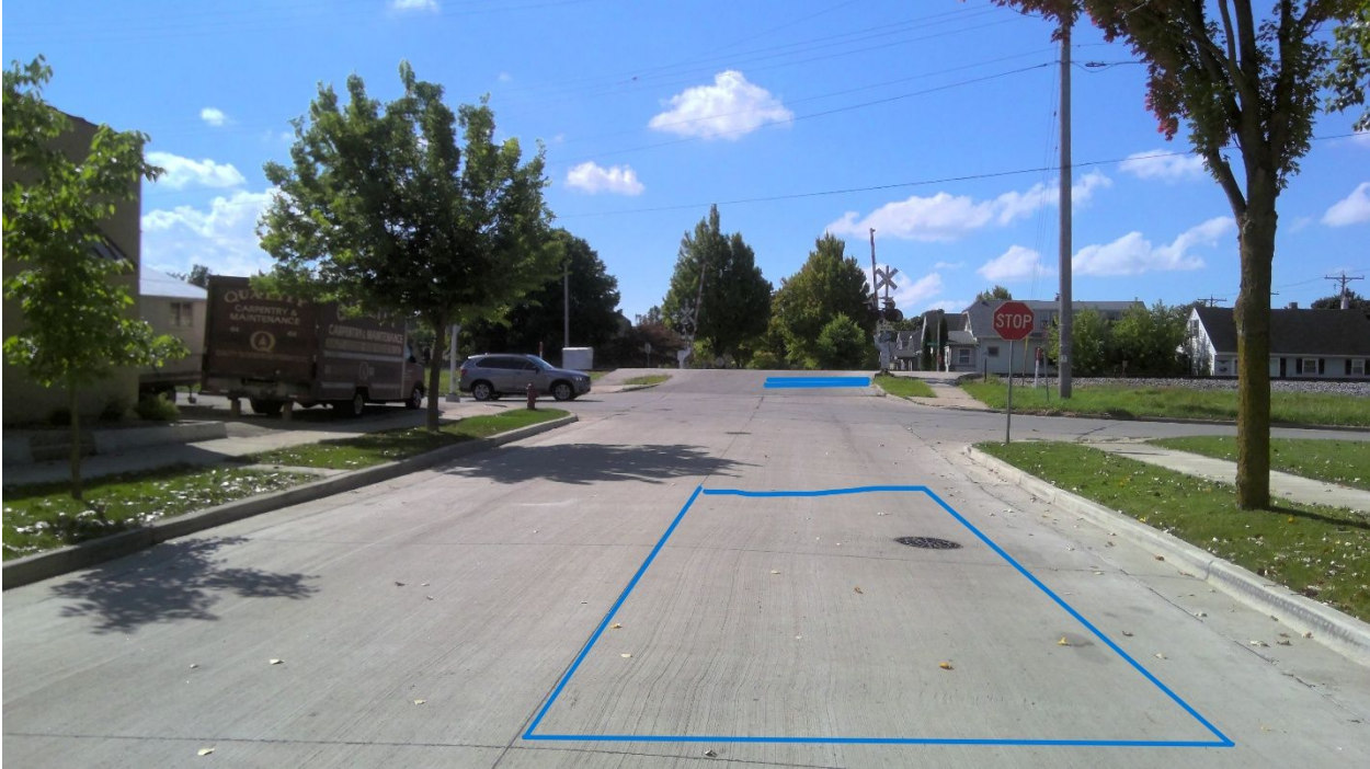
Missing pavement markings and stop lines
