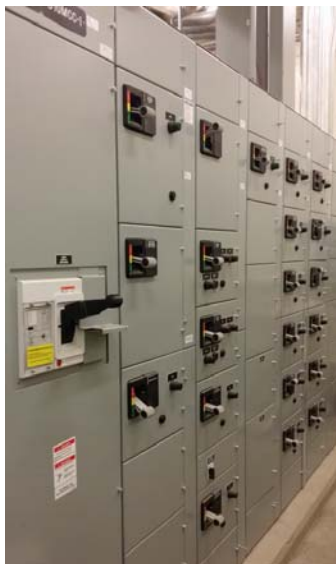
Energenecs Supplied MCC at Eau Claire WWTP
