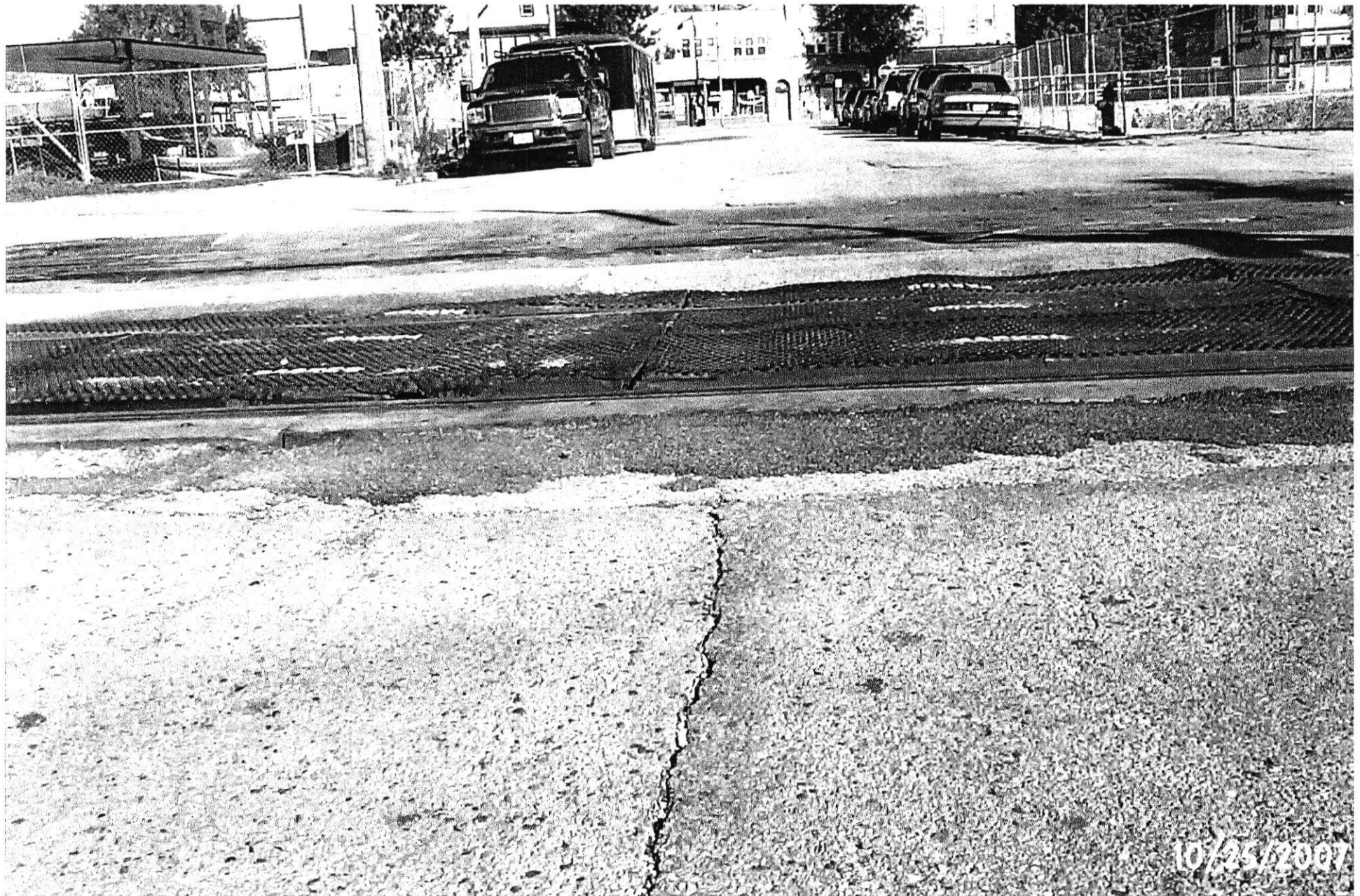
Picture taken by Brian Block on 10-25-07 of the UPRR At-Grade crossing at S 80 St. U.S DOT crossing No. 177247V. Standing south of tracks looking north
