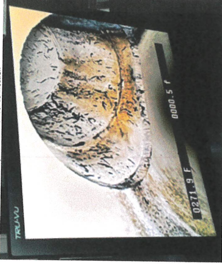
Figure 1: View from the sanitary main of the riser connection
