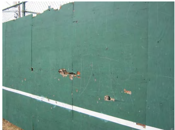
The tennis ball return wall is damaged
