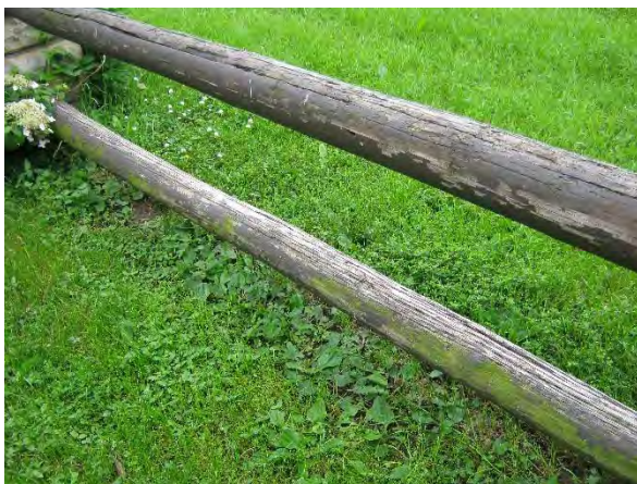
Worn trellis beams
