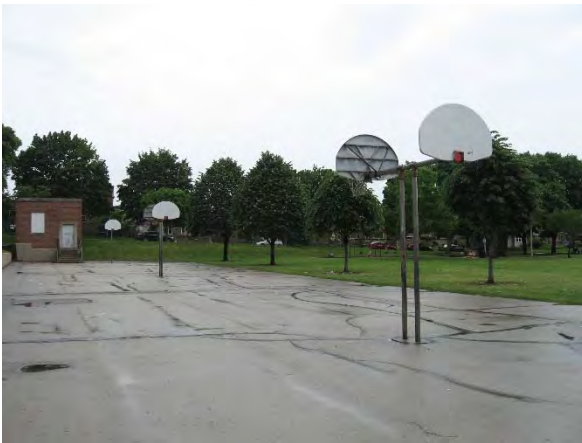
Basketball court paint is faded
