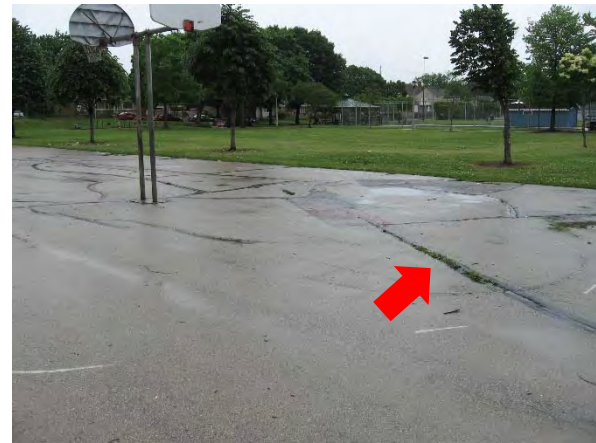
Weeds growing through cracks in court
