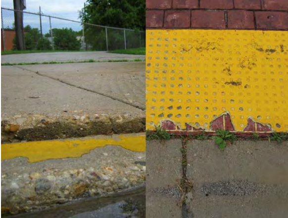
Issues at curb ramps
