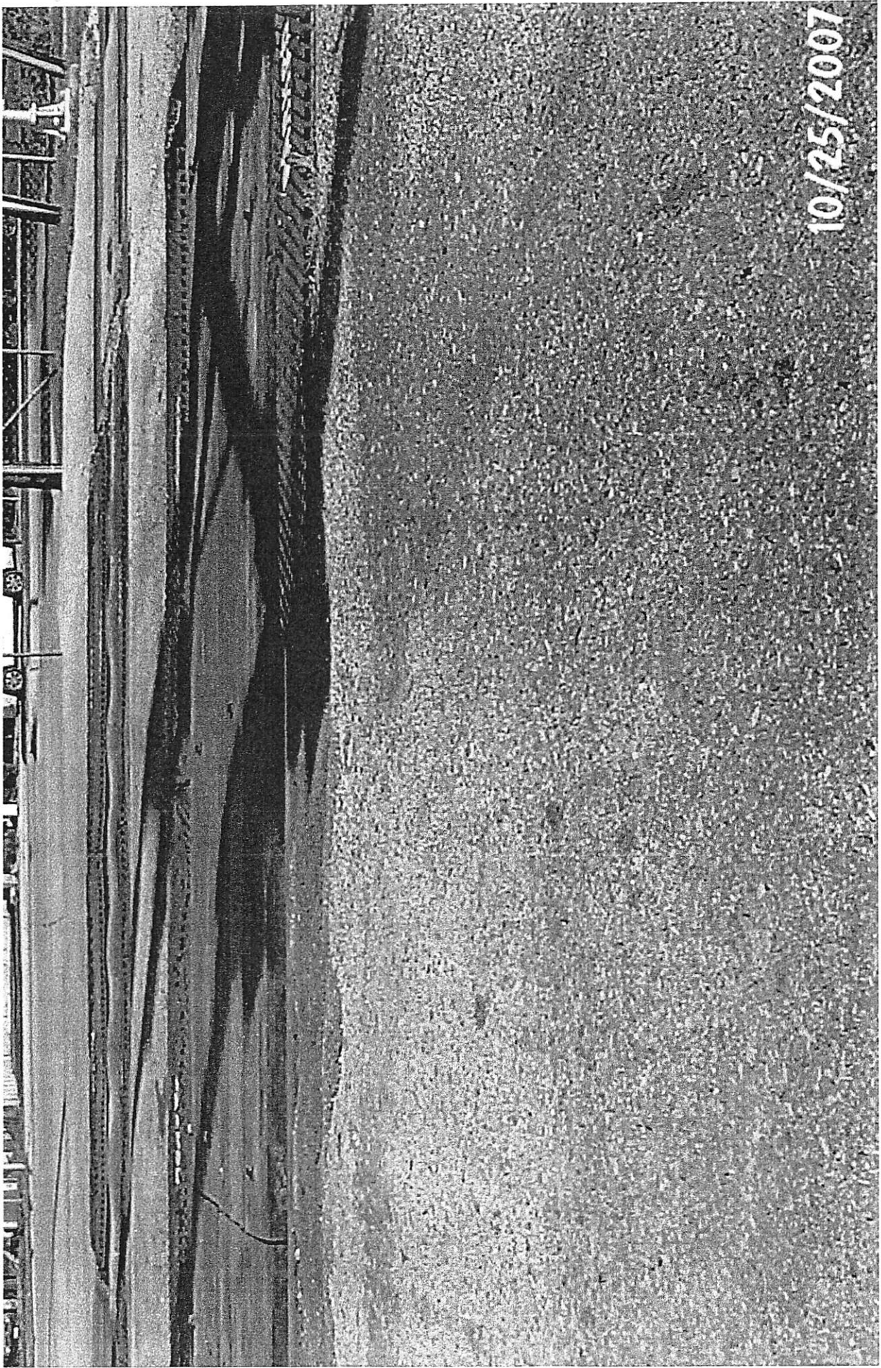
Block on 10-25-07 of the UPRR At-Grade crossing at S 82 St. U.S DOT crossing south of tracks looking north
