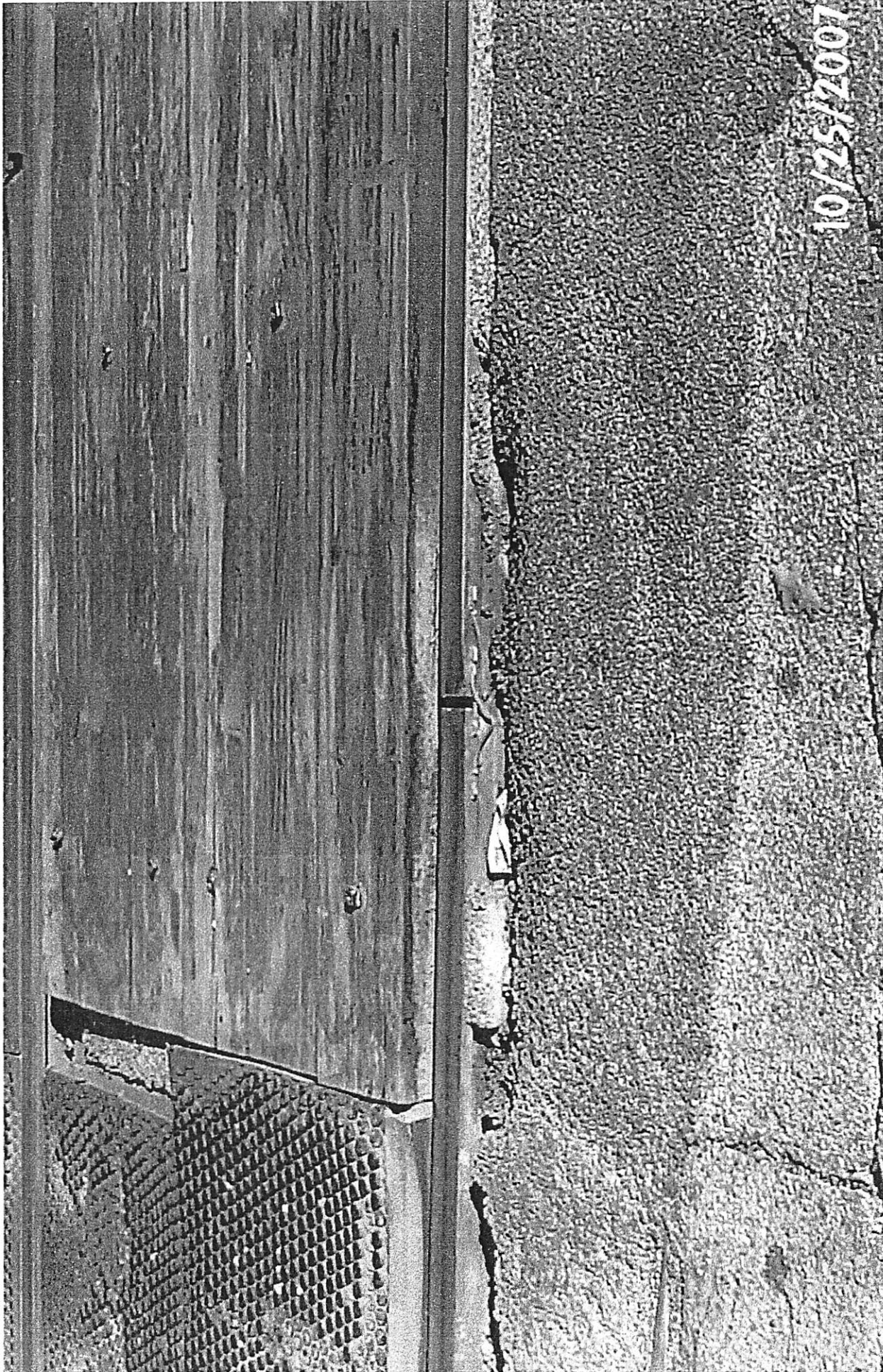
Block on 10-25-07 of the UPRR At-Grade crossing at S 82 St. U.S DOT crossing south of tracks looking north
