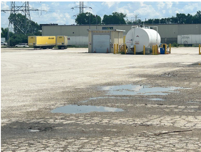
Asphalt in poor condition
