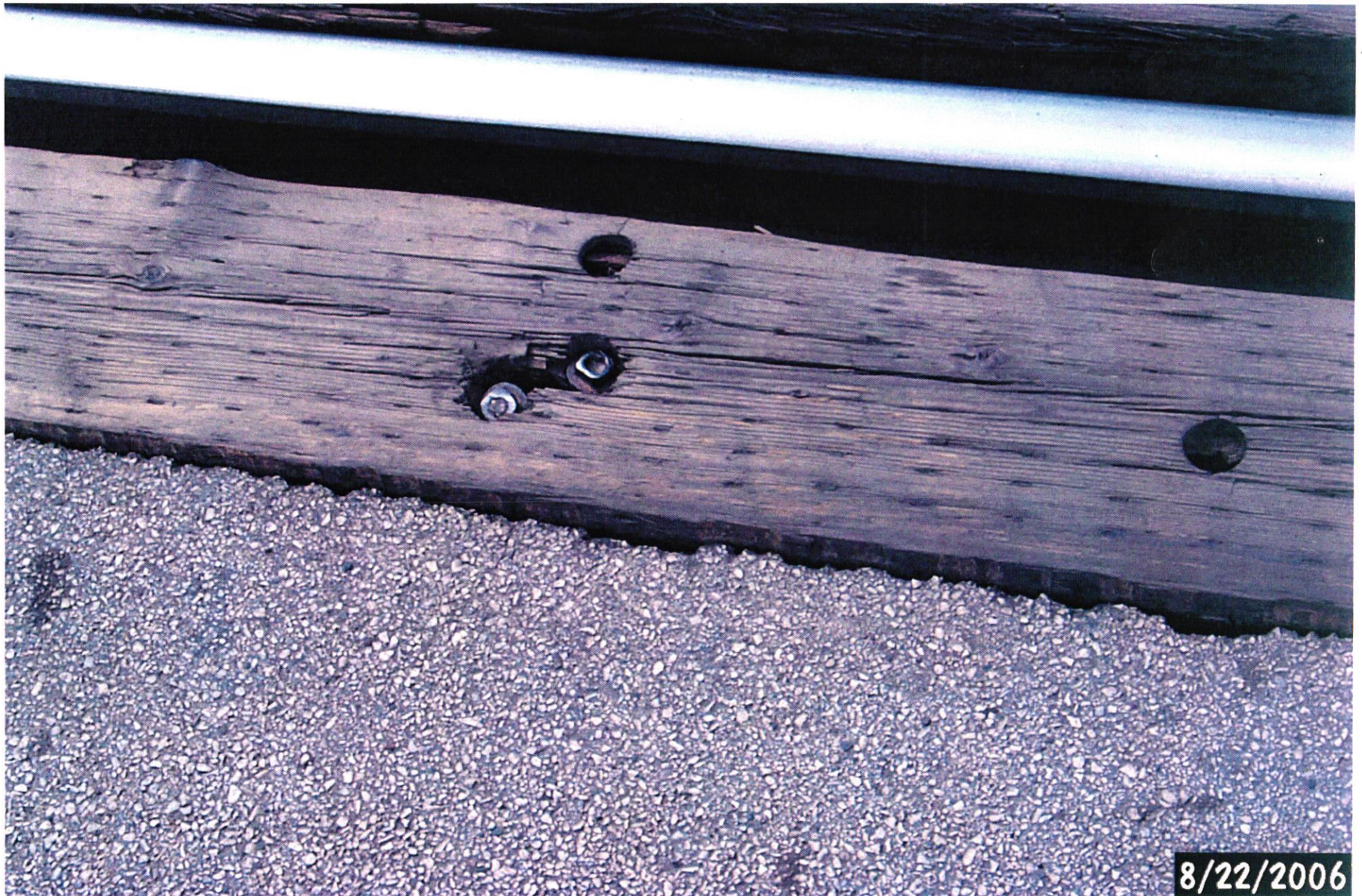
Picture taken by Brian Block on 08-22-06 of the Union Pacific at grade crossing in S 55 St-north tracks, rotted wood that rocks upward when traffic drives over.
