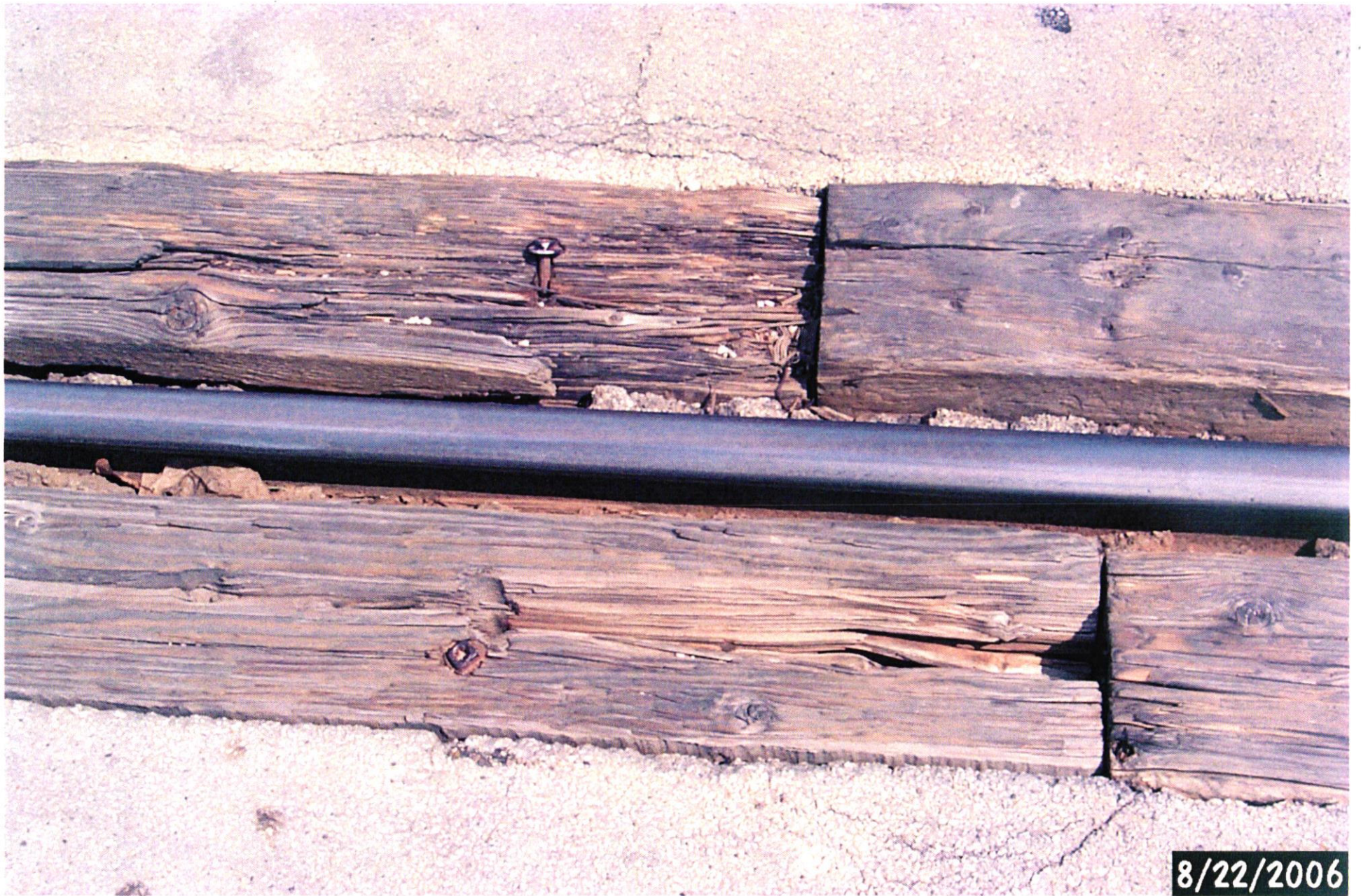
Picture taken by Brian Block on 08-22-06 of the Union Pacific at grade crossing in S 57 St-north tracks.
