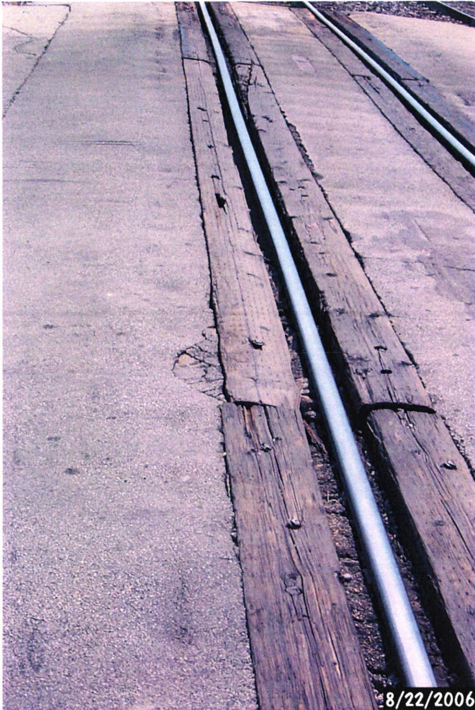
Picture taken by Brian Block on 08-22-06 of the Union Pacific at grade crossing in S 55 St-north tracks, rotted wood that rocks upward when traffic drives over.
