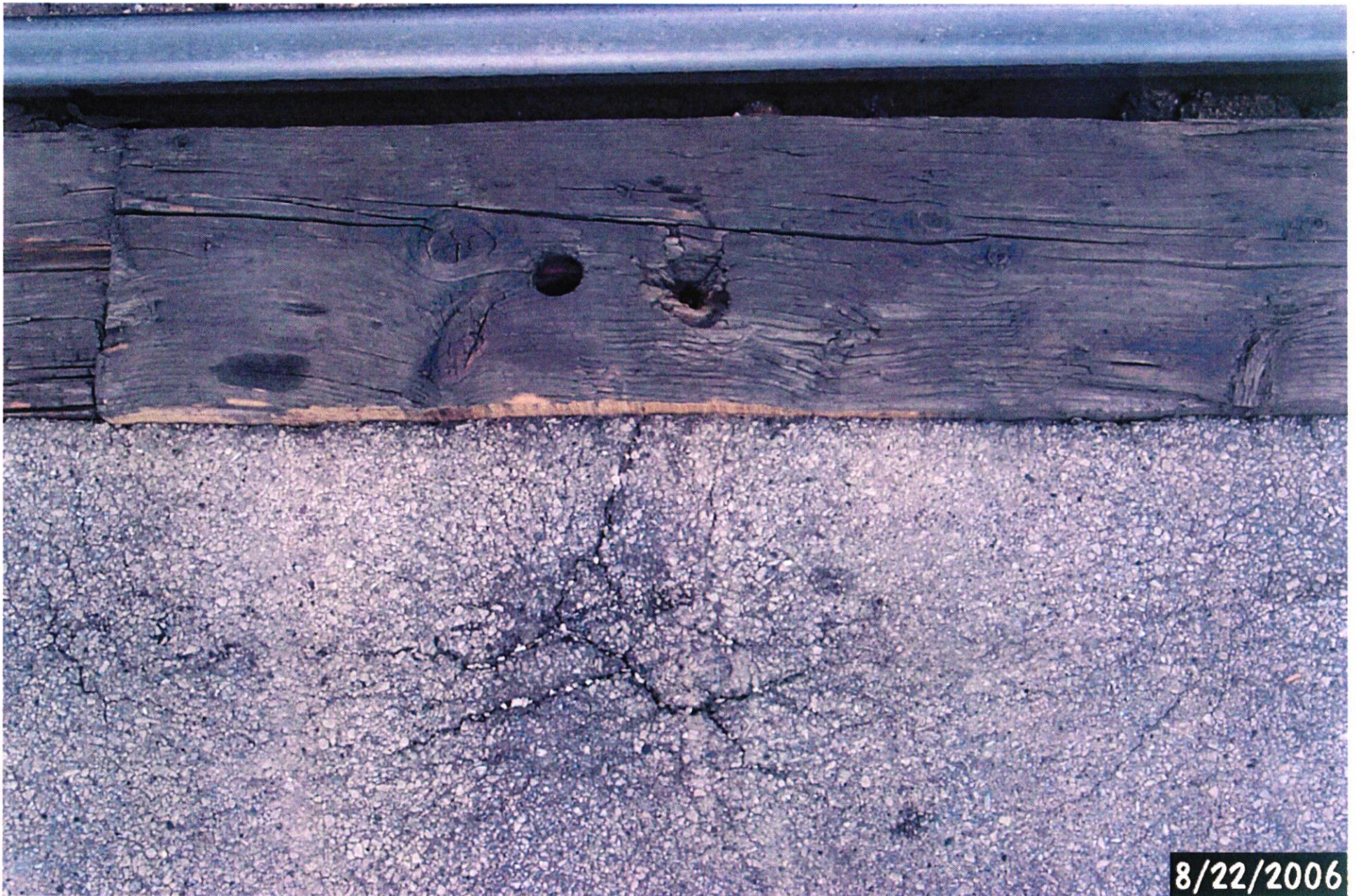
Picture taken by Brian Block on 08-22-06 of the Union Pacific at grade crossing in S 57 St-south tracks. Fasteners not holding wood rocks with vehicles traveling over it.
